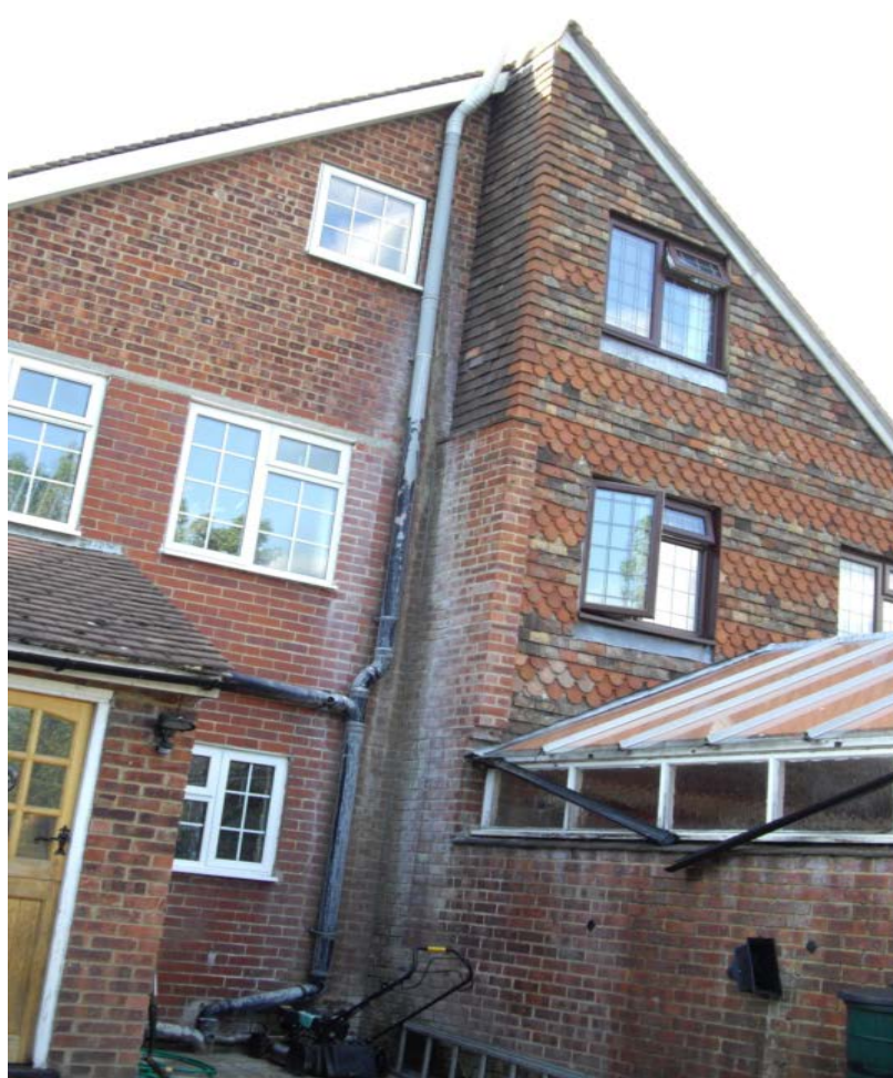
Figure 9. External view from neighbours side (NW) of rear addition/conservatory prior to rebuild works showing the high level windows recessed from the cavity wall.
